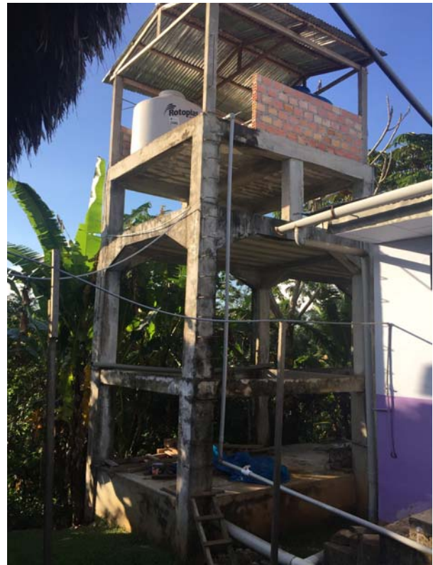
Fig. 1. Water tower in Nauta, Peru. Fiberglass tanks can be seen at the top, and the main transmission line can be seen exiting the bottom right of the photo.
